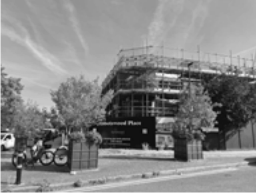
Abbotswood Place squeezed into the plot of a demolished 1950s corner house
